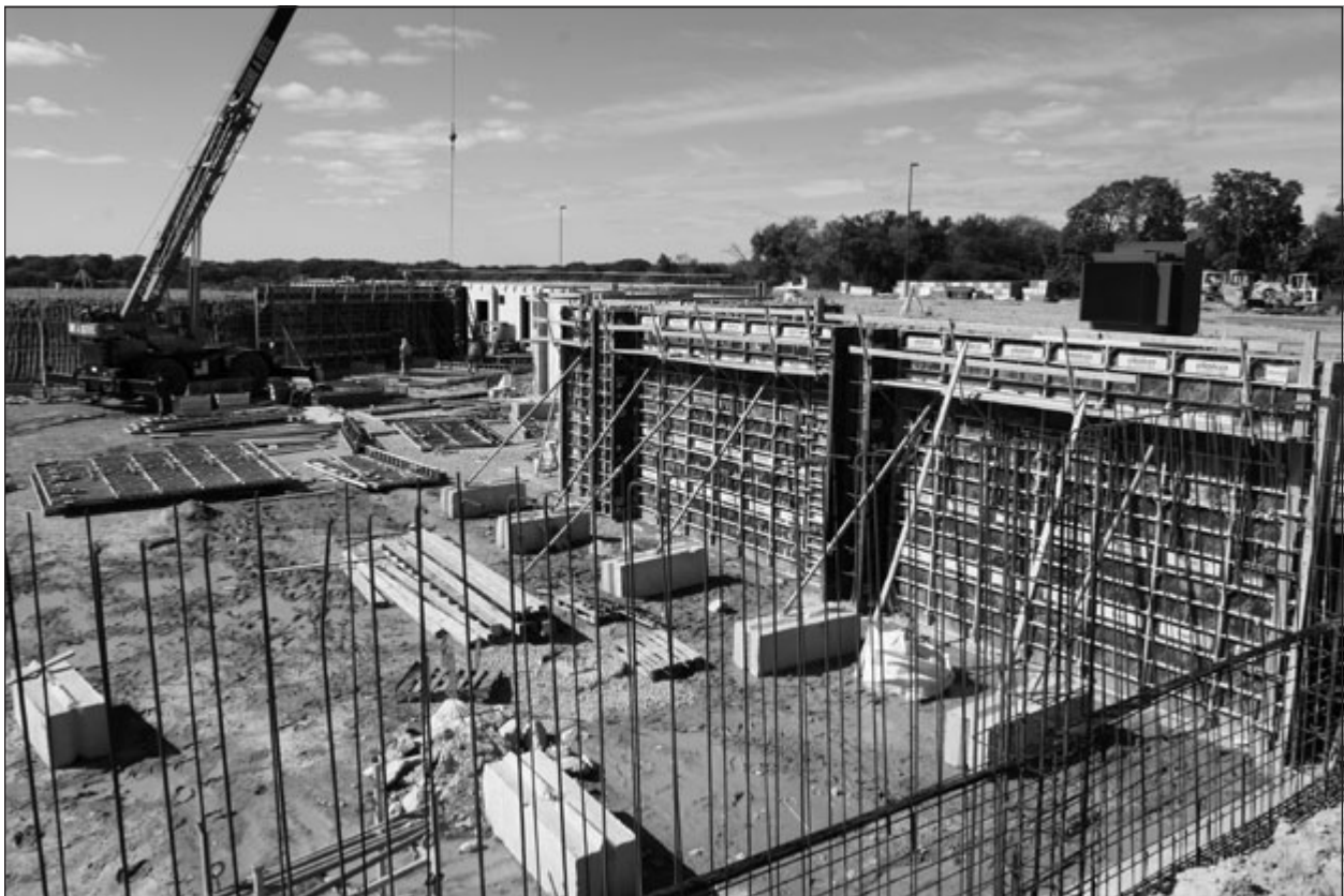
The well-organized worksite and good housekeeping aided productivity of the foundation wall installation for the Wheaton Bible Church.
