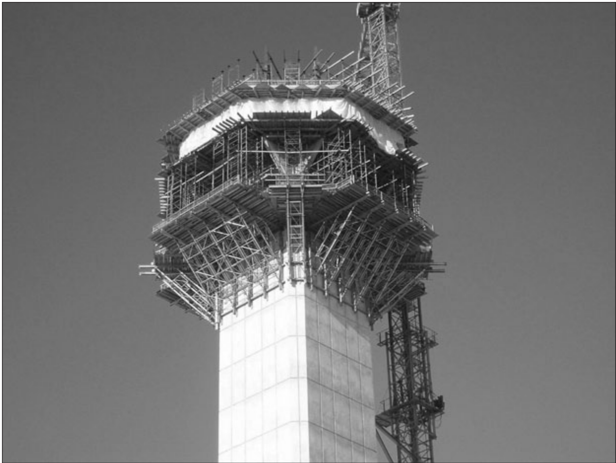
Concrete form work (a concrete cost line item) and access scaffolding (a general condition cost line item) must be planned together for maximum productivity and safety. STUFORM® and JUMPFORM concrete wall form work along with 20K® shoring towers were supported by custom-designed support frames for construction of the air traffic control tower at Washington Dulles Airport, VA. Photo courtesy of Harsco Infrastructure.
